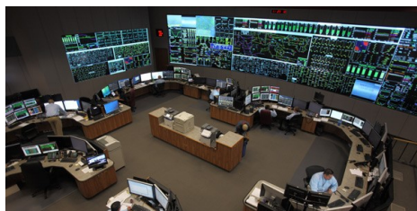
PJM control room | PJM
